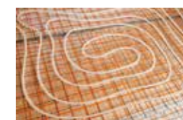
Floor heating loop
